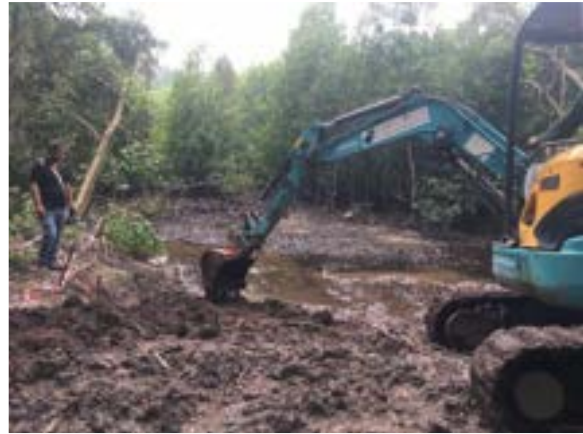
Fig. 15. Regrading of soil to lower the ground level for more areas to be inundated.
