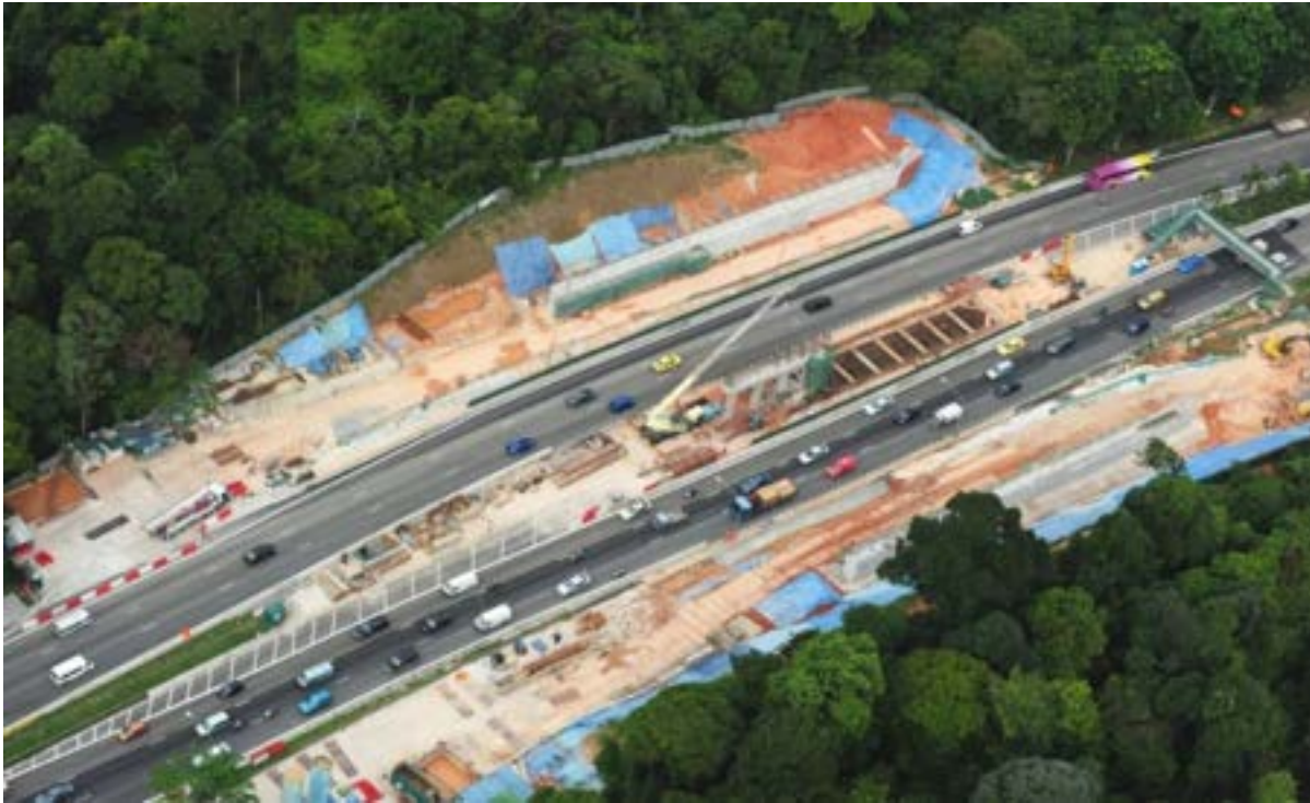
Fig. 2. The traffic flow along the BKE was maintained throughout the construction phase, while the inconvenience for the commuters along BKE was minimised.
