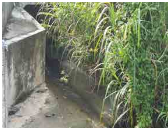
Fig. 3. Freshwater inputs entering the mangrove forest via the bund for overflow from the pond and lined drains.
