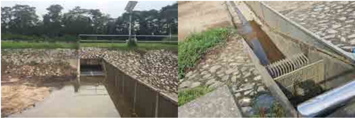
Figs. 8. A filtration system at the start of drain channels into the mangrove area.
