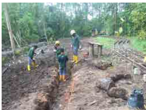
Fig. 16. Trenching of channels to bring in seawater for more areas to be inundated during high tide.
