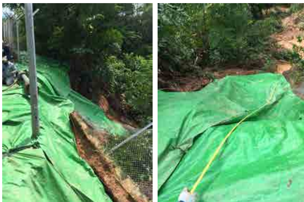
Figs. 3. Large canvas sheets were laid over to prevent the saturation of soil, which might lead to further slope failure.
