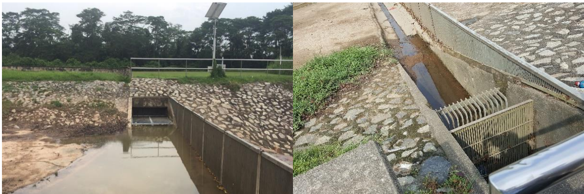
Figs. 8. A filtration system at the start of drain channels into the mangrove area.
