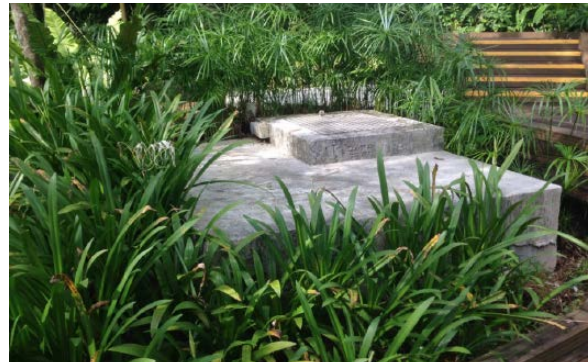
Water Bulk Meter
