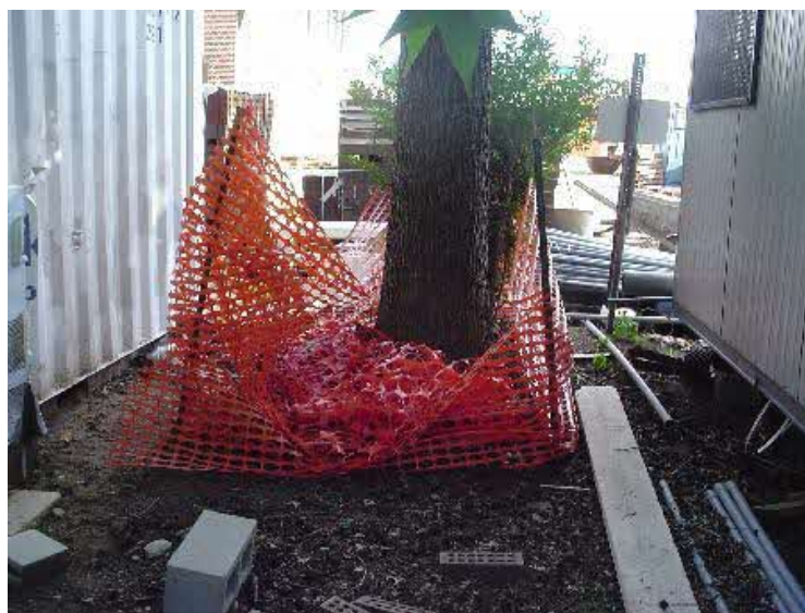
Figure 7: Inappropriate installation/maintenance of TPZ during construction.
