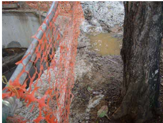
Figure 5: Construction cement deposited at tree base.
