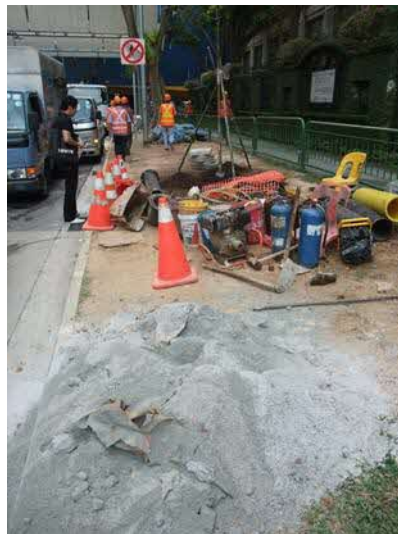
Figure 1: Construction material and heavy machinery are prohibited within the TPZ
