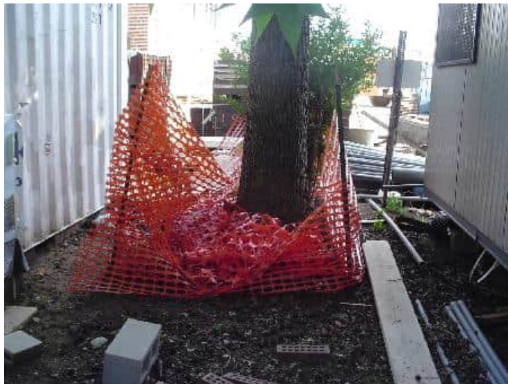
Figure 8: Inappropriate installation/maintenance of TPZ during construction
