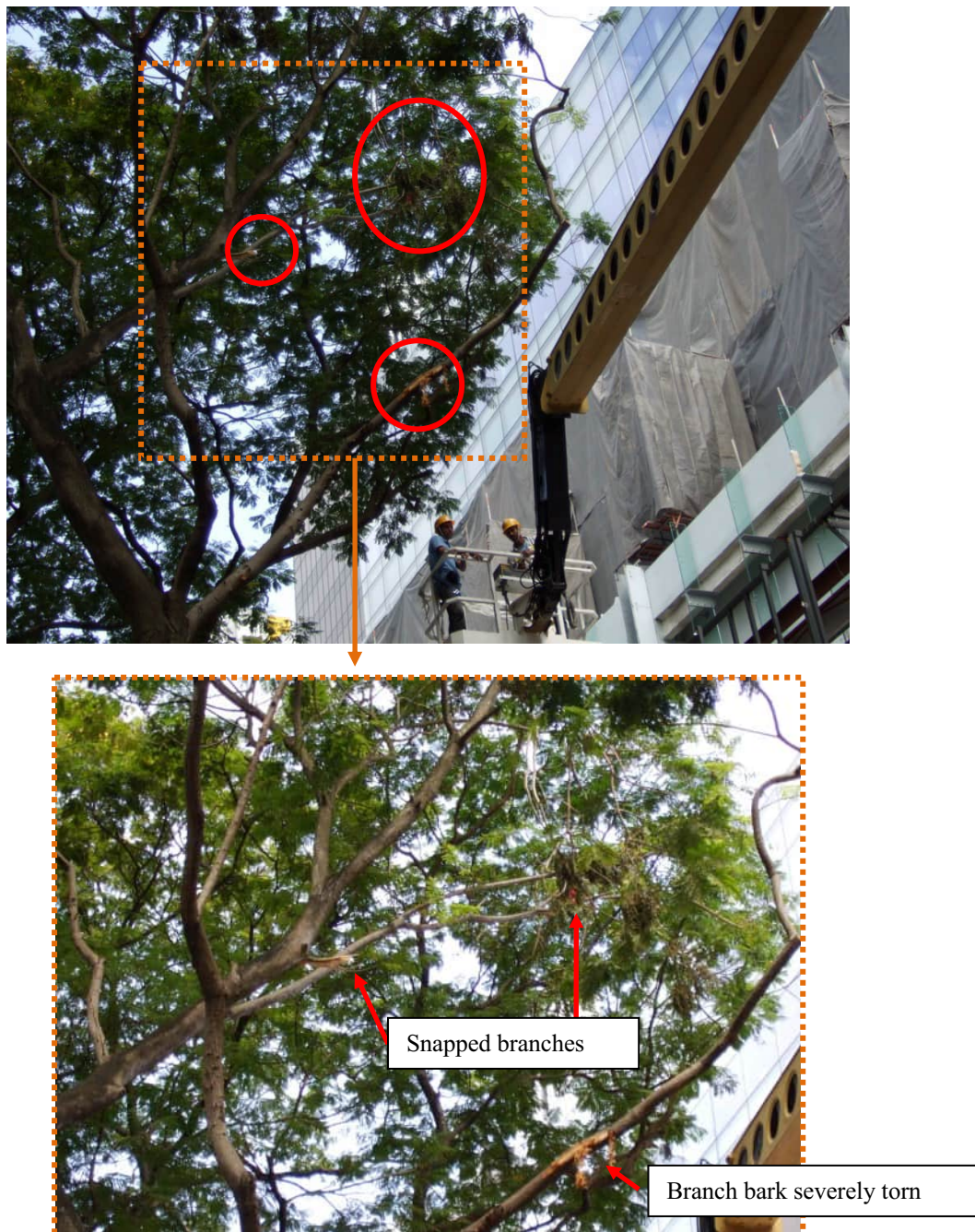
Figure 9: Tree branches were severed due to the negligence of the crane operator
