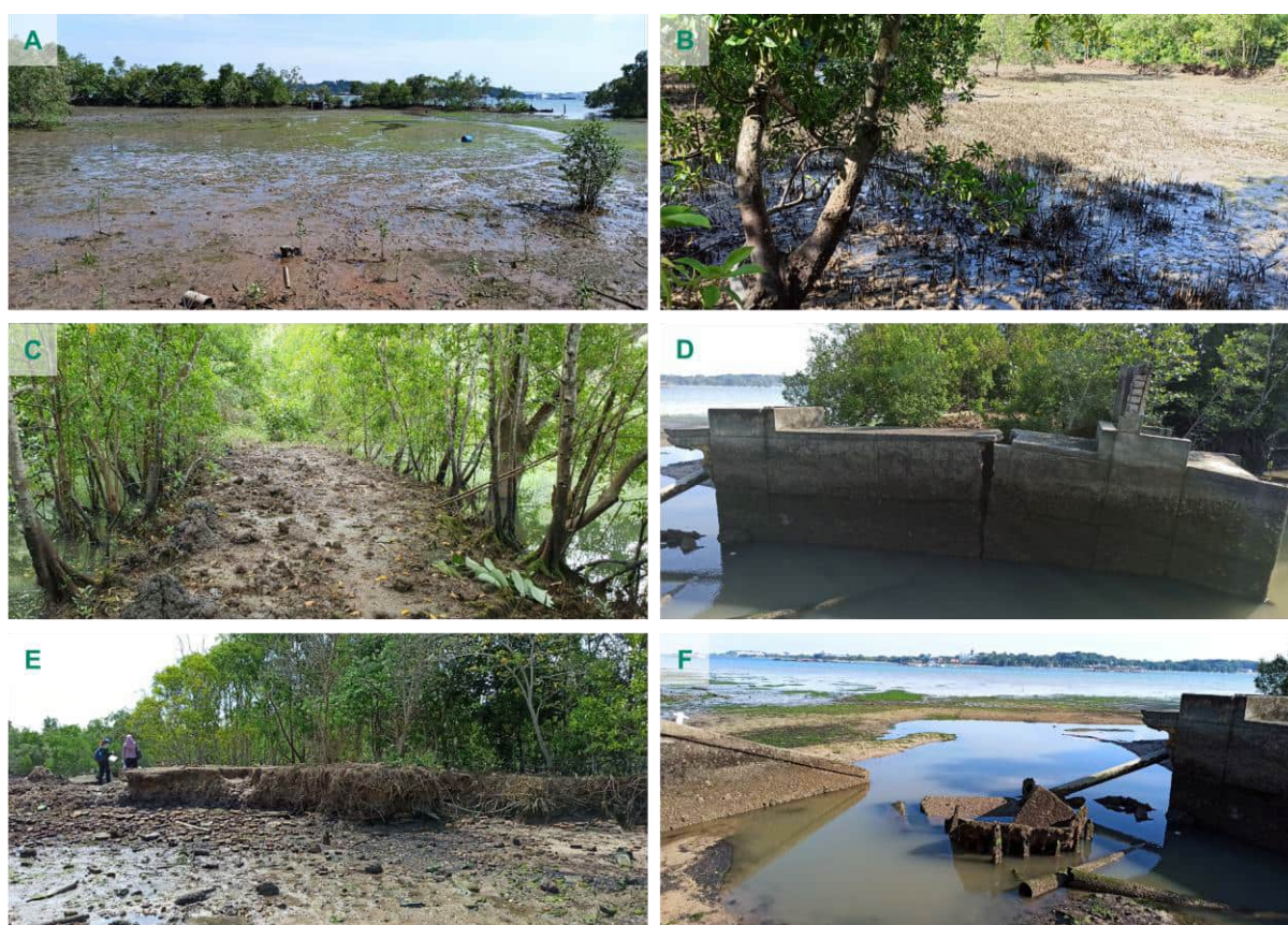
Figure 3-3 Photos of existing site conditions (A) Pond 3 at low tide, (B) Mangroves growing within Pond 1, (C) Mangroves growing along the bunds between Pond 1 and Pond 2, (D) Broken sluice gate at south of Pond 1, (E) Severe erosion of bunds near the opening of Pond 3, and (F) An opening formed between two sluice gates at the south of Pond 1 and Pond 2.
