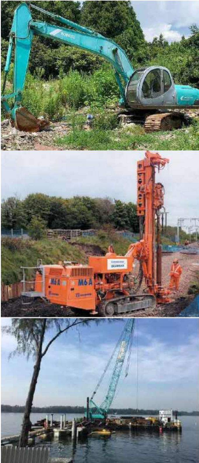
Figure 2.3 Construction equipment types to be used for the development (Top: for trimming of seabed; Middle: for micro piling; Bottom: for marine piling)
