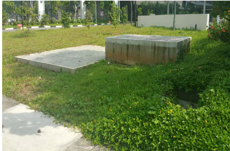
Bulk Water Meter
