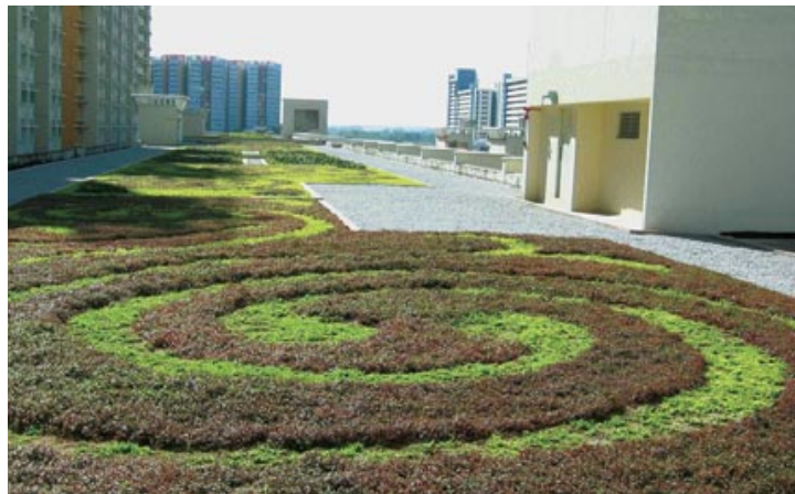
NParks partnered HDB on this pilot rooftop greening project, at Edgefield Plains in Punggol.
