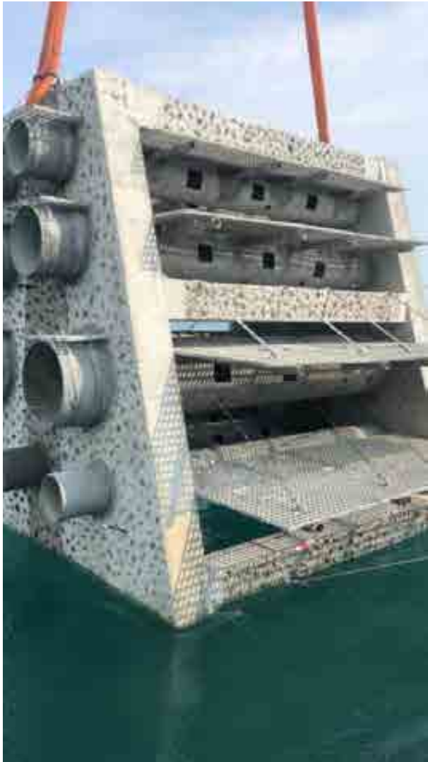
Fig. 2. Top section of artificial reef structure being lowered into the sea. (Photo credit: Srirangam Santosh Kumar)
