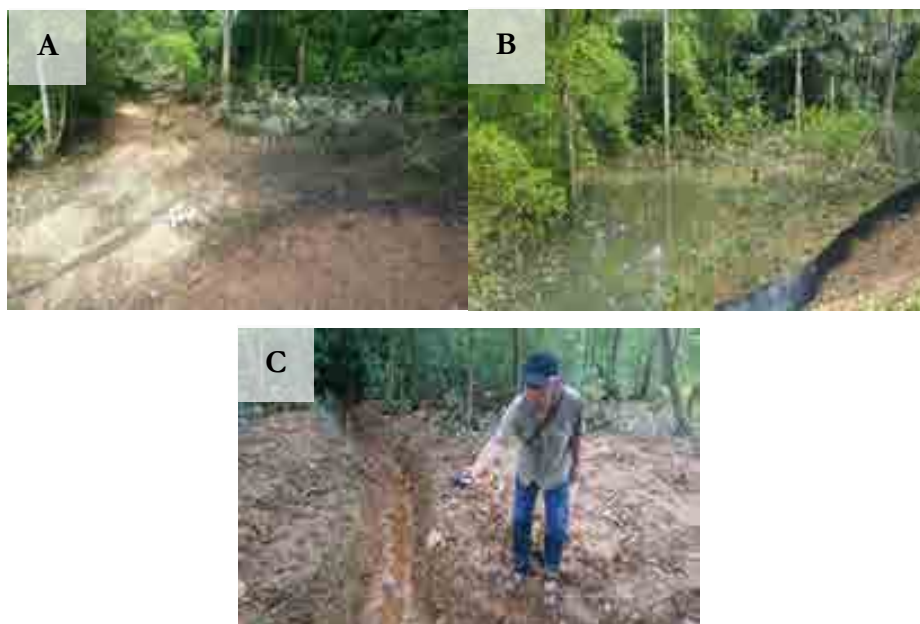
Figs. 7. (A) Excavated channels in mangrove; (B) Monitoring of tidal flow at the channels; (C) Mapping of the excavated channels.
