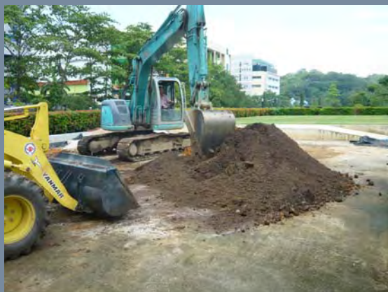
Figure 1. Mixing ASM offsite results in a uniform mix, avoiding subsequent drainage problems.
