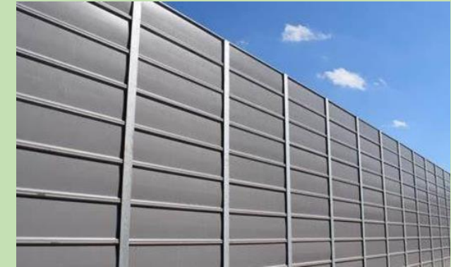
Conventional noise barrier
